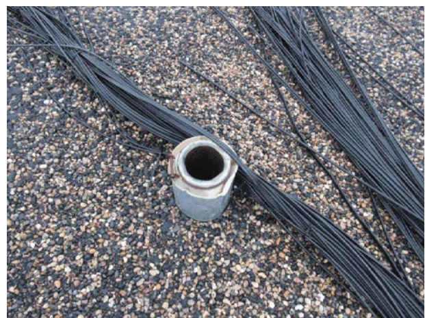
Minor vent damage
