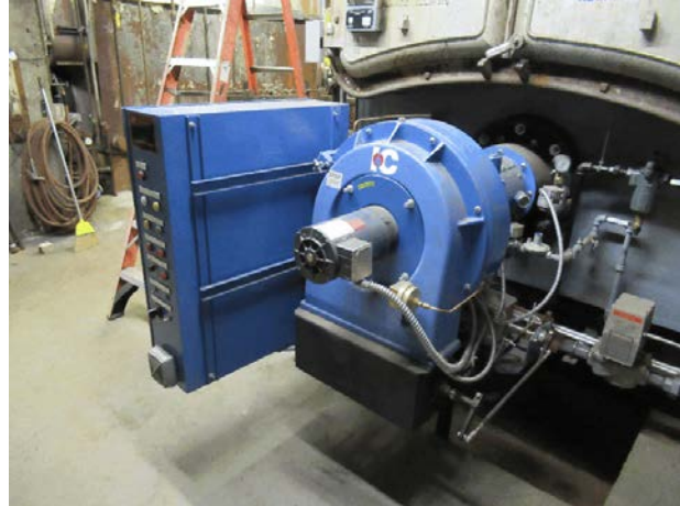
Burner and controls
