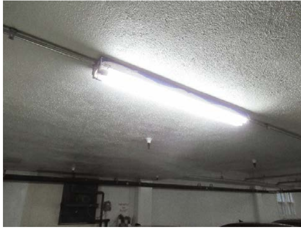
Overview of light fixture
