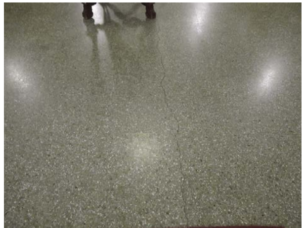
Terrazzo floor crack
