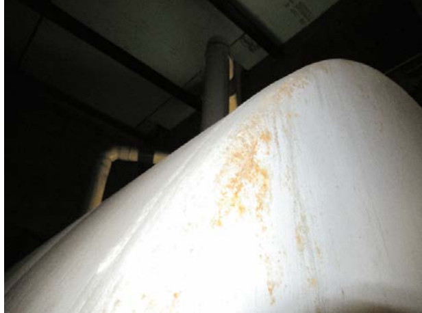
Minor surface corrosion
