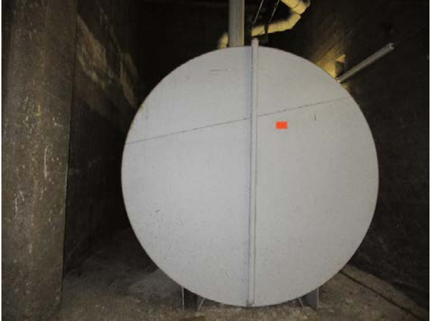
Overview of fuel storage tank
