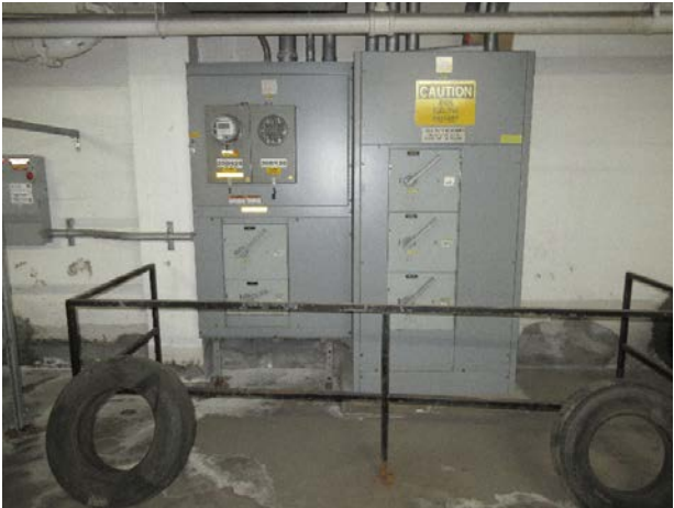
Overview of primary switchgear
