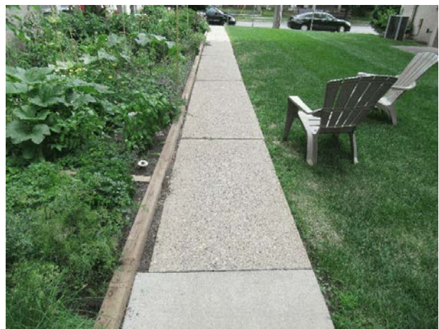
Sidewalk overview with surface pitting
