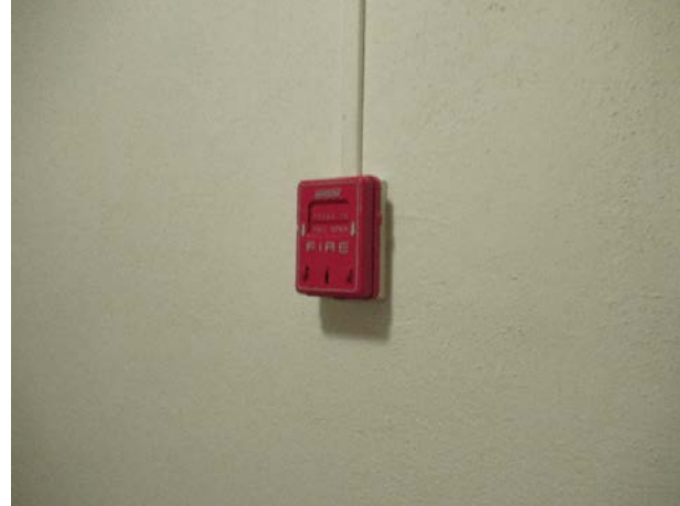
Emergency device – pull station
