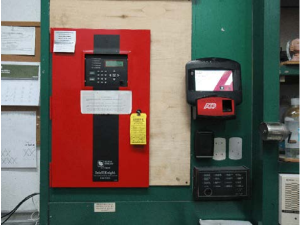
Life safety system control panel
