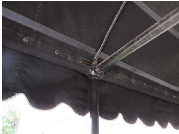
Minor frame corrosion
