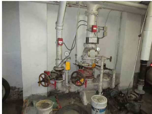
Fire suppression system inlet piping and valves
