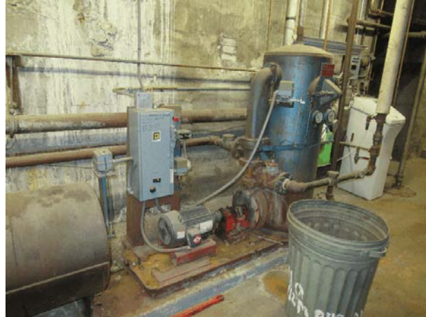
Condensate return system
