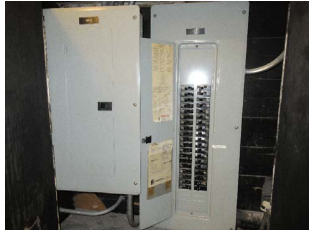
Overview of hallway circuit breaker panel
