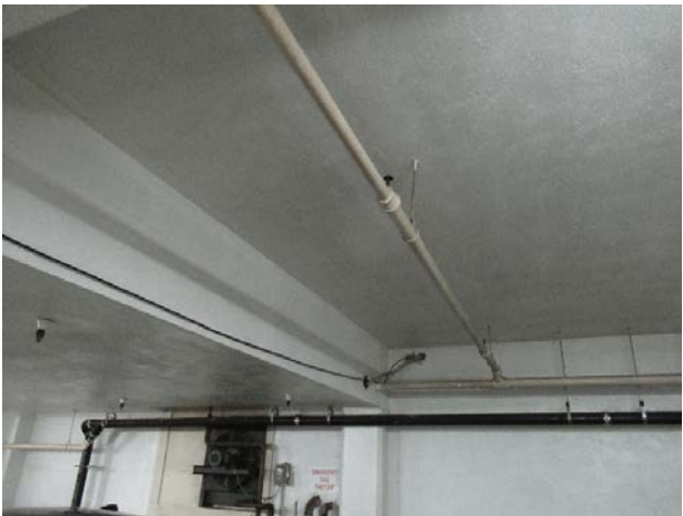
Fire suppression system piping and sprinkler head
