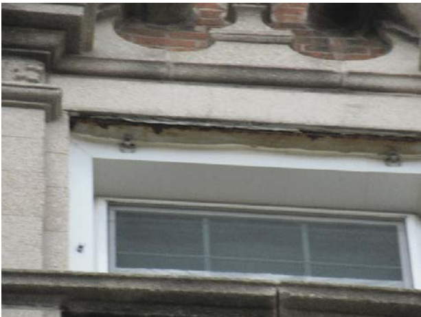
Lintel with significant corrosion
