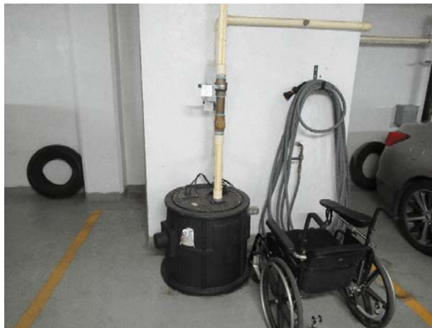
Garage sump pumps
