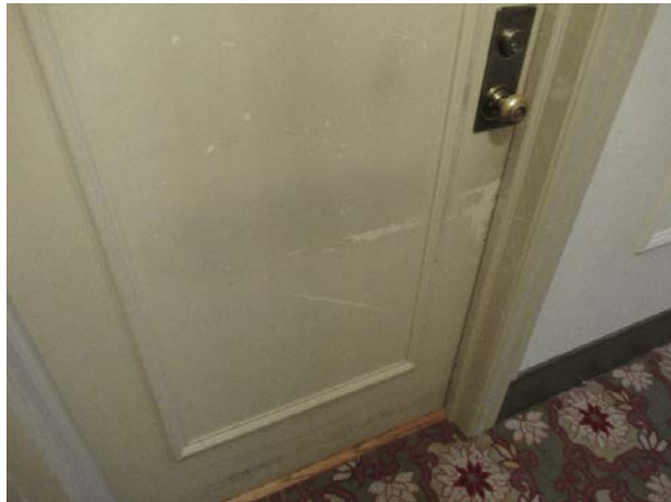
Significant scuffs at entry doors
