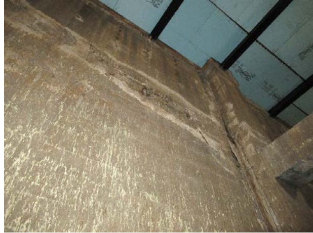
Prior water stains
