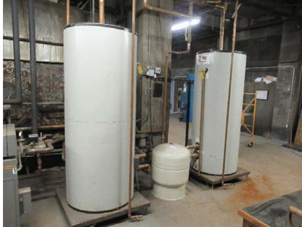
Domestic hot water storage tanks
