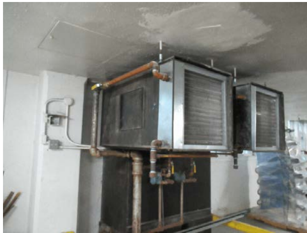
Overview of unit heaters
