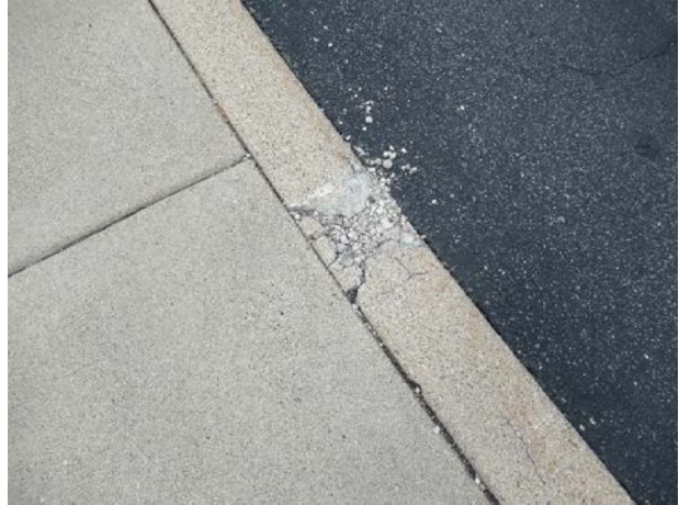
Concrete curb deterioration
