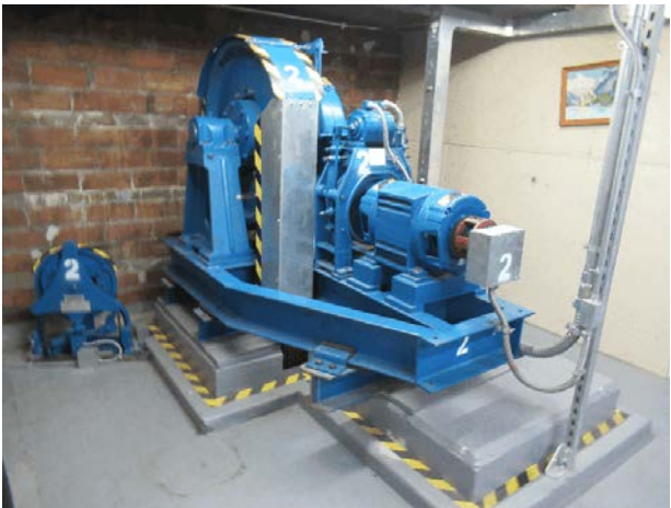
Passenger elevator hoist and motor
