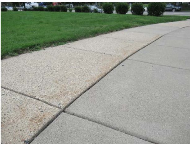
Sidewalk overview with surface pitting
