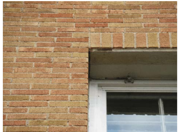
Mortar deterioration above lintel
