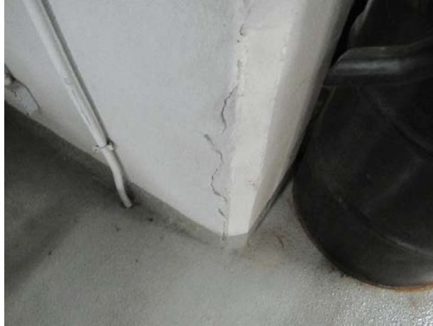
Deterioration of wall concrete
