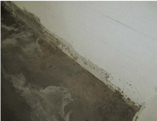
Concrete deterioration at lower walls
