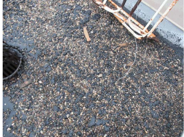
Blistering – condition is a result of the expansion of air beneath the bituminous
