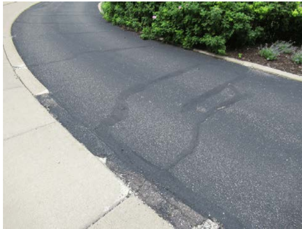
Transverse cracks with prior repairs
