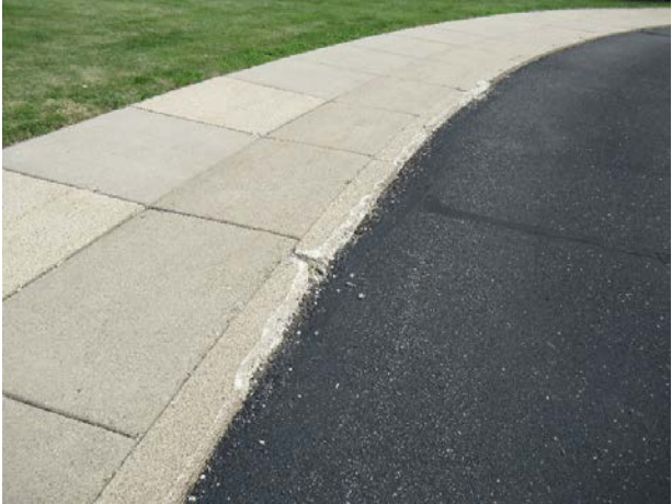
Curb overview with concrete deterioration
