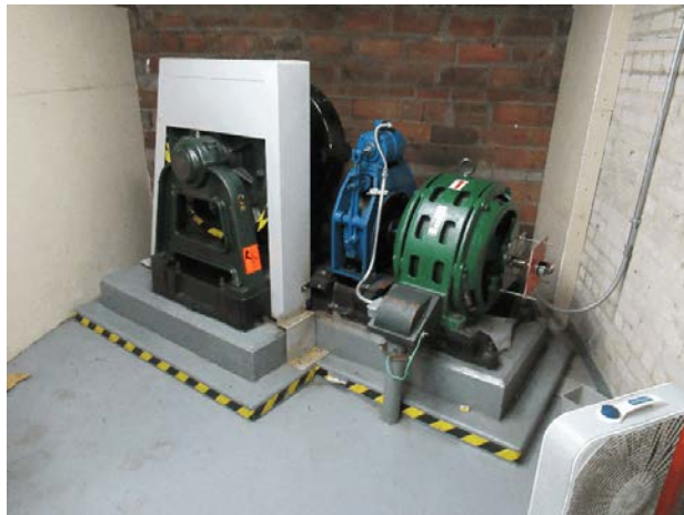
Freight elevator hoist and motor
