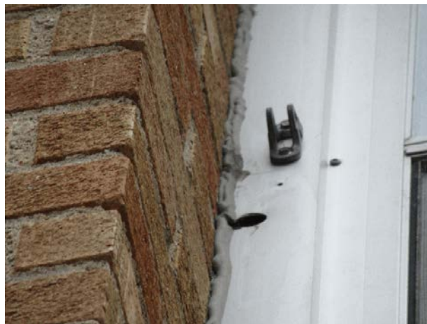
Frame damage with prior sealant repair
