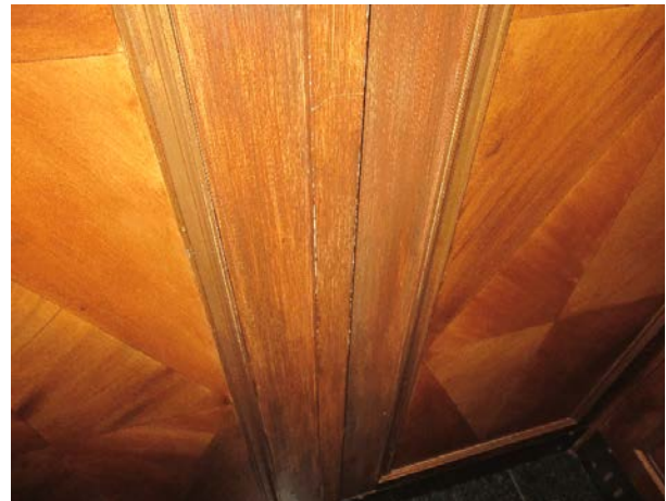
Wood walls with finish deterioration
