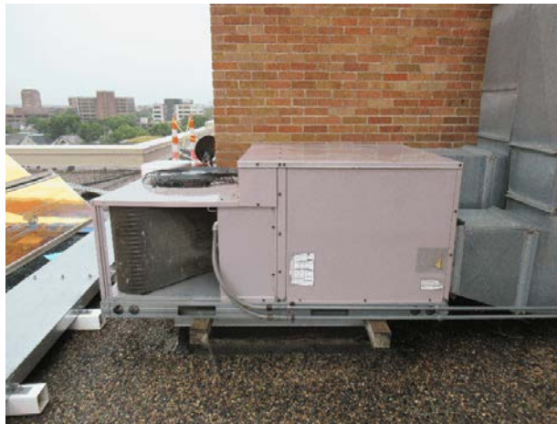
Rooftop air handling unit
