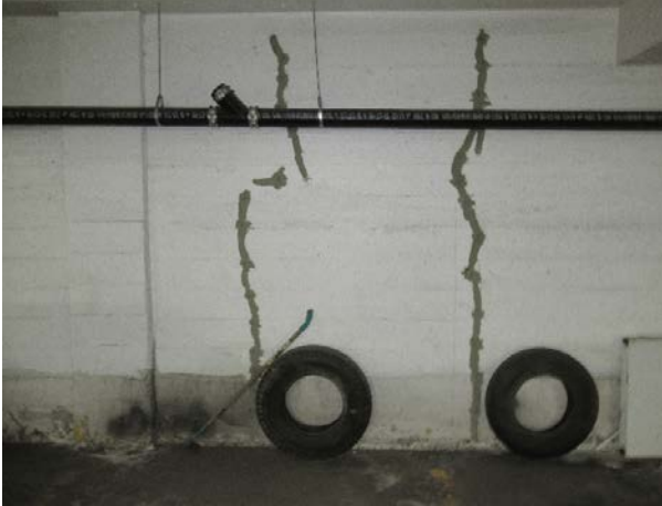
Prior wall crack repairs
