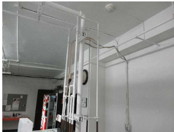
Electrical wiring for laundry machines uses extension cords run externally to wall outlets
