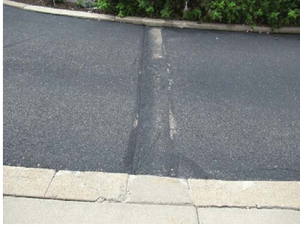
Transverse cracks with prior repairs
