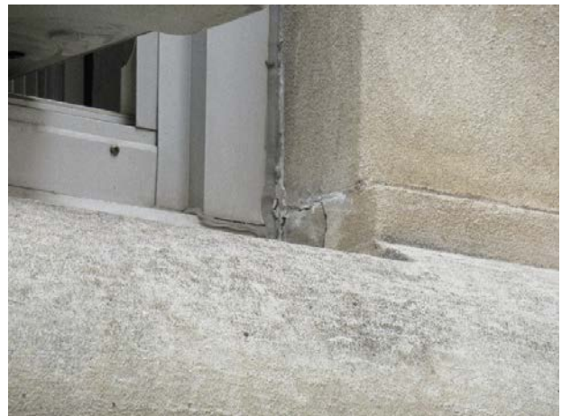
Crack at prior concrete repair
