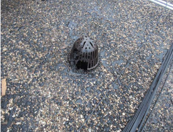
Damage of roof drain
