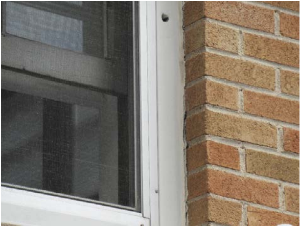
Window sealant deterioration
