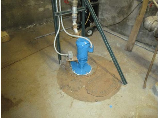
Boiler room sump pump
