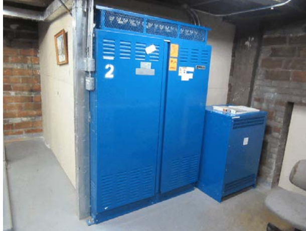
Passenger elevator controls
